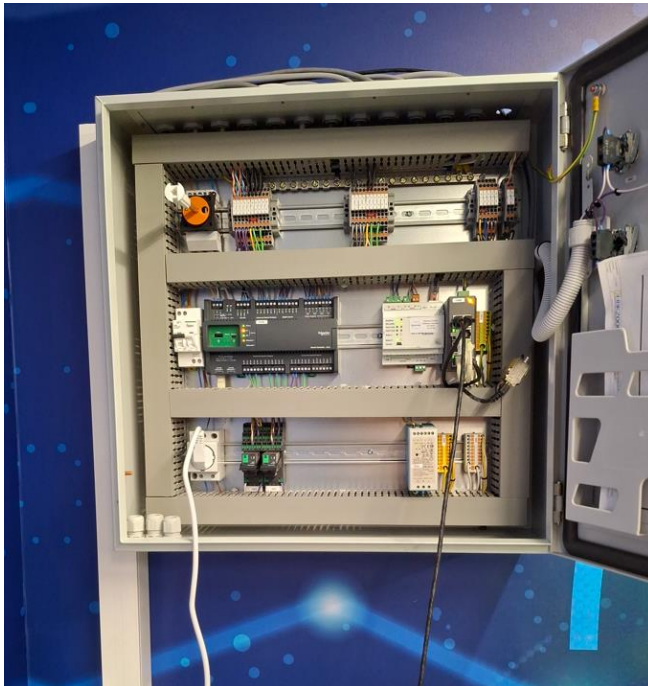
Figure 17: Control panel for the sensors in the cooling loop.
