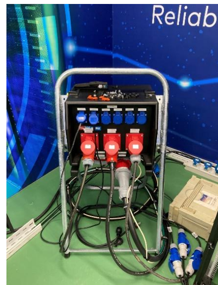
Figure 6: Battery energy storage.
