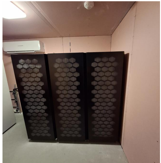
Figure 5: Battery energy storage.
