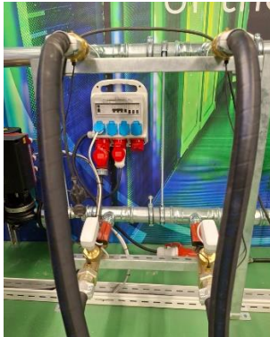
Figure 7: Compact Power Distribution Unit.
