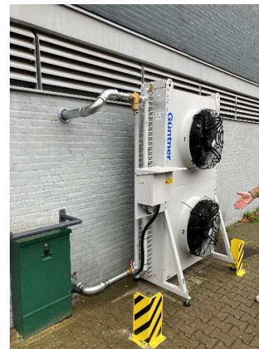
Figure 8: Air-cooled dry cooler.
