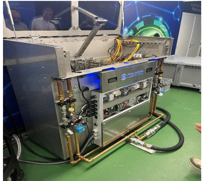
Figure 14: Asperitas PNC immersion tank.
